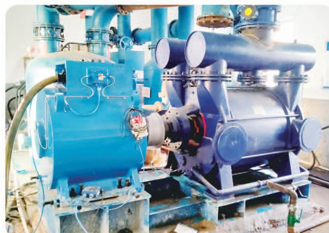
Gas drainage pump
